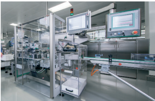
REA VeriMax integrated into a production plant
