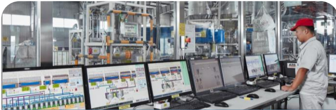
Control Systems, PLCs, HMIs & Industrial PCs
