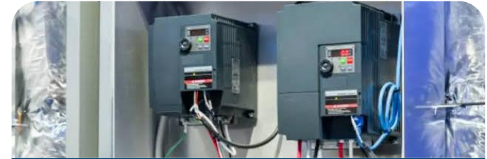
Electrical Components, Connectivity & Control Panels
