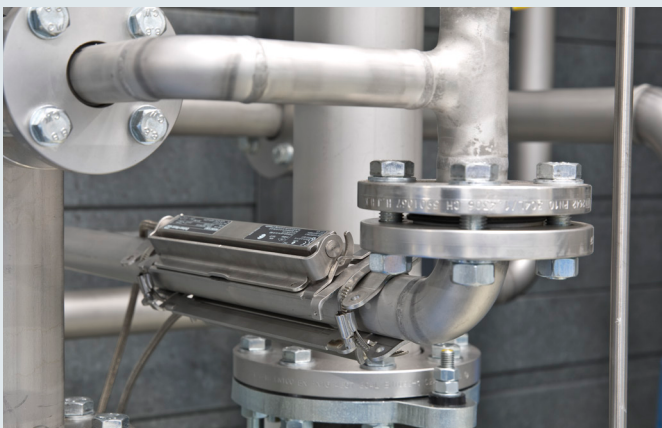
Replacement measurements for defective flowmeters
