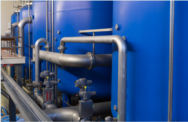
Cooling and process water (utilities)
