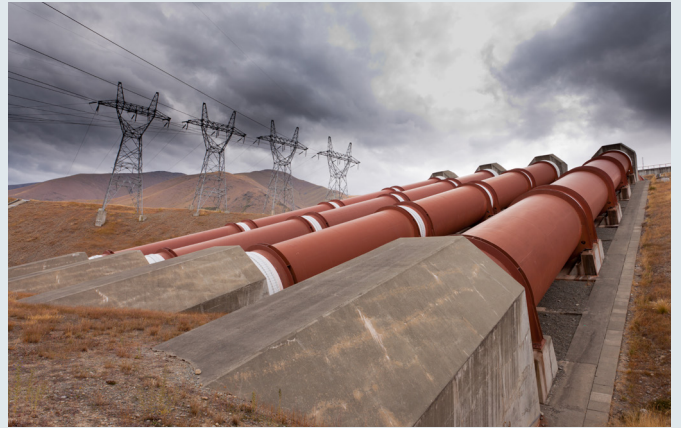
Water in penstocks (energy/power plant industry)
