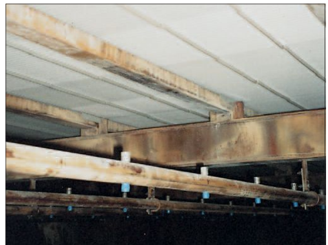
Installed LTV 400 in a flue-gas desulphurization plant
