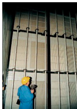
Installed LTH 100 in a flue-gas desulphurization plant
