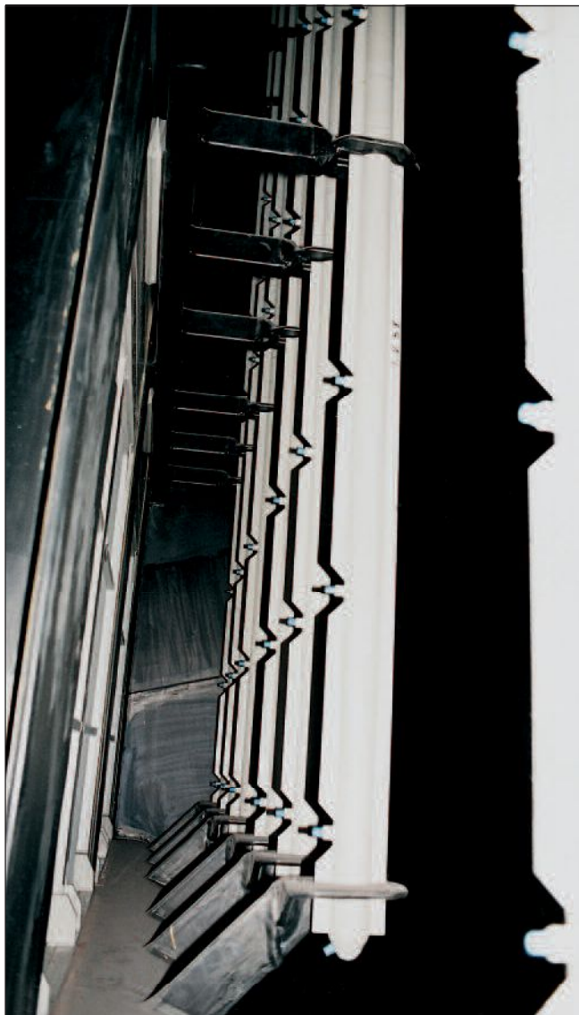
Nozzle spray system
