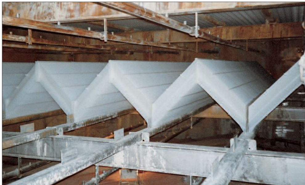
LTV 110.33.-B in a wash tower
