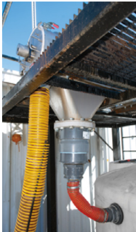
Oversized grain solids exit through downspouting into an enclosed container. Recovered liquid (sour mash) gravity feeds through the center discharge, is stored and added to subsequent fermentation batches.
