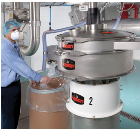
Downstream of the spray dryer, a Kason screener removes oversize particles. Because of the company’s expertise in spray drying, “overs” (spout at right) comprise a small percentage of the total batch.
