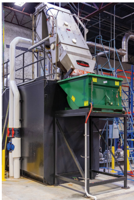
CROSS-FLO Sieve removes solids from 28,000 gal (106,000 l) per day of TGD Cuts’ wastewater before it enters the municipal wastewater system.
