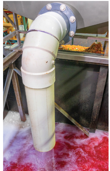
Screened wastewater is pumped to the municipal wastewater plant in compliance with accepted levels of total suspended solids.
