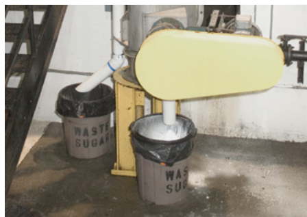
Oversize material falls through a 4 in. (102 mm) diameter chute and drops into a tailings bin.
