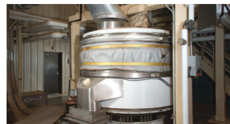
An 84 in. (2125 mm) diameter circular fluid bed dryer, clad with insulation blanket, dries almonds to moisture content between 4.5 and 5.5 percent. Throughput rate is 22,000 lb (9,979 kg/h) per hour.
