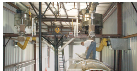
Two 60 in. (1524 mm) diameter Kason VIBROSCREEN screeners are used to load trucks with sugar at the SBS Sparta facility.
