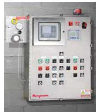
Programmable controls allow plant personnel to automatically start, stop, slow, speed-up, delay, advance or cycle equipment functions.
