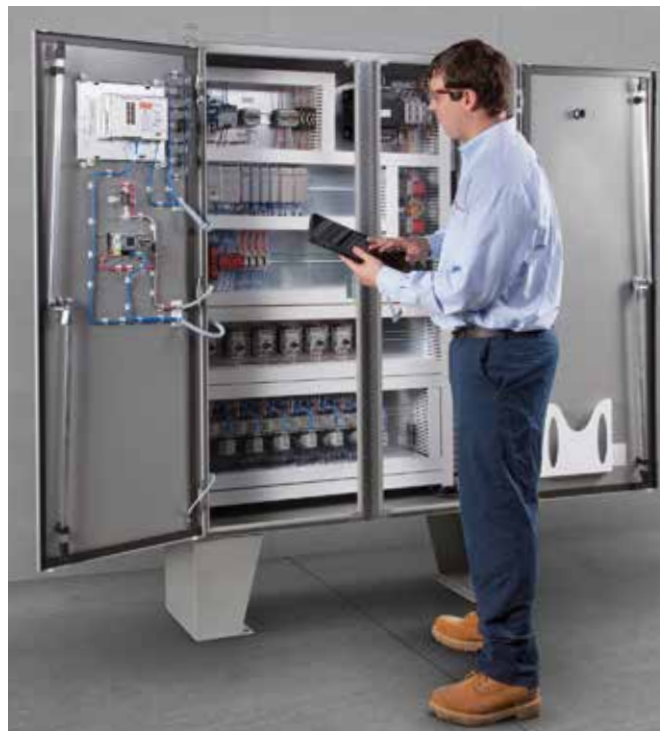
Plant personnel can download programs to start, stop, slow, speed-up, delay, advance or cycle equipment functions.
