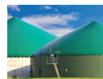
Biogasanlagen Bio gas plants
