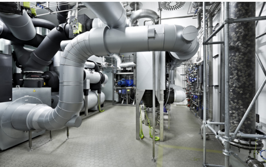
Technical area of a Coating unit with nitrogen circuit and solvent condensation
