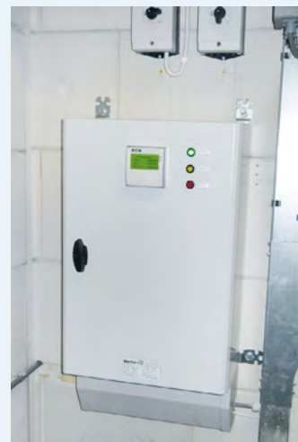
Heating Group International switch panel
