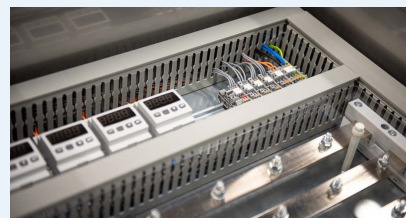
Stainless steel 316 cabinet housing divided into 4 electrical groups
