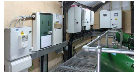
Electrical control room
