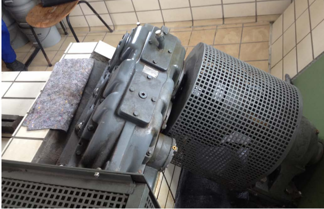
Before: existing (third-party) gear unit on the worm shaft in Kleinsteinbach
