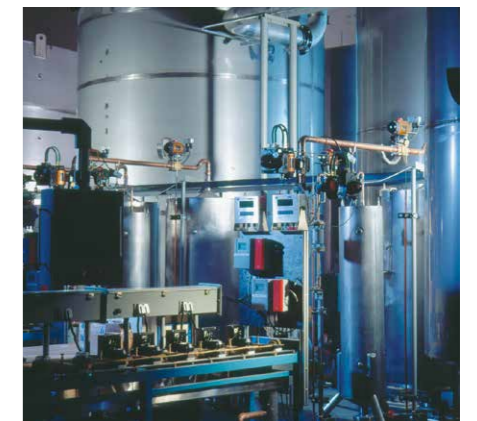
Test stand and innovation center of Badger Meter
