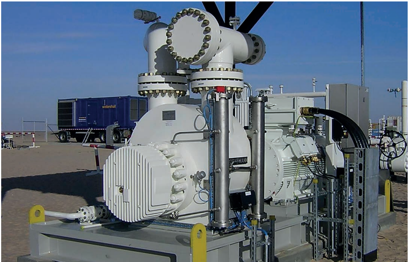
Multiphase „Boosting in Libya“
