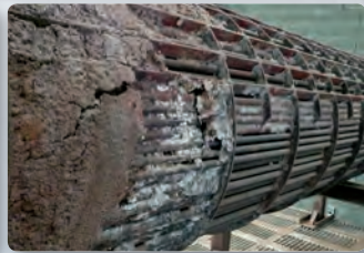
AFTER THERMAL CLEANING: 5% DUST, EASY TO REMOVE
