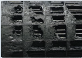
BEFORE THERMAL CLEANING: 100% POLLUTION
