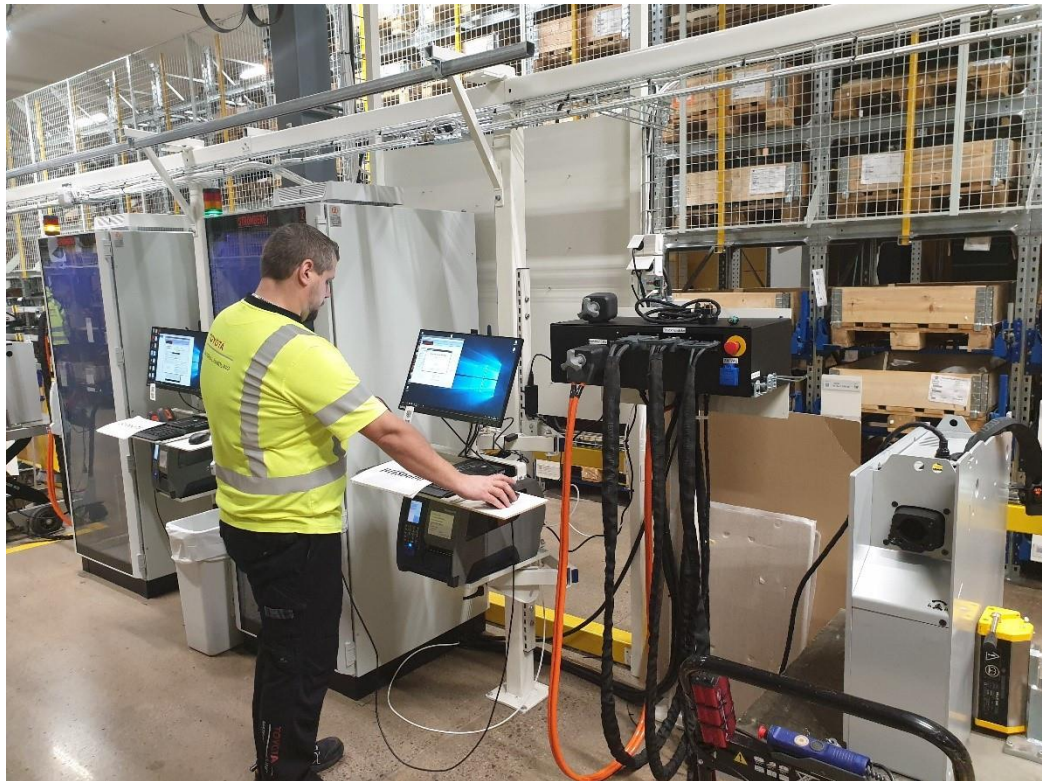
Figure 4 The operator initiates the charging and test sequence
