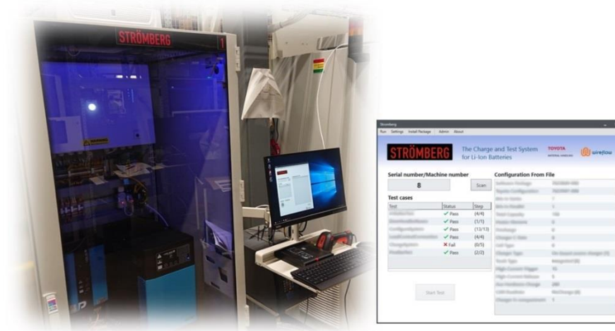
Figure 2 Cabinet, PC and Operator control panel
