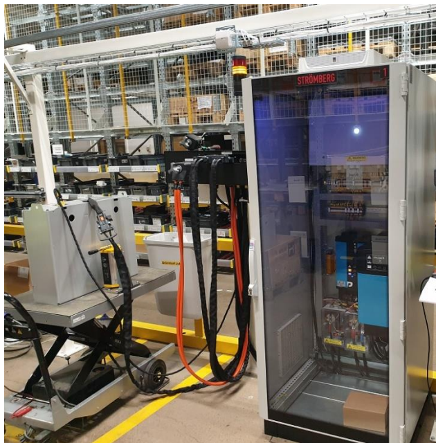
Figure 3 A battery being charged and tested by the cabinet
